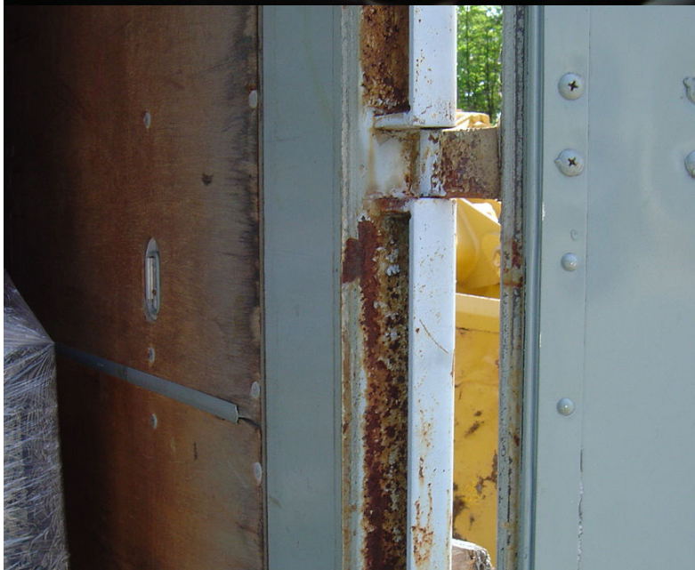
The storage container corrodes but not the equipment inside Intercept packaging.
